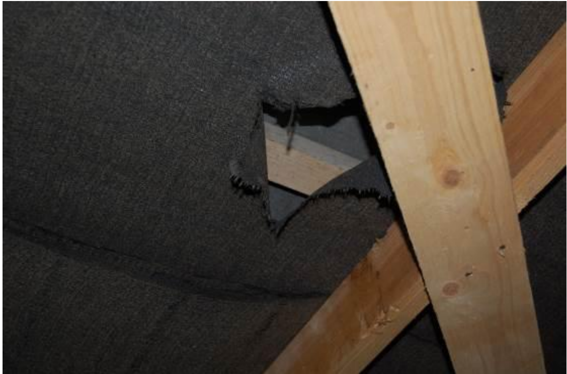
Photo 3 Small Hole in Sarking Felt to be Repaired
