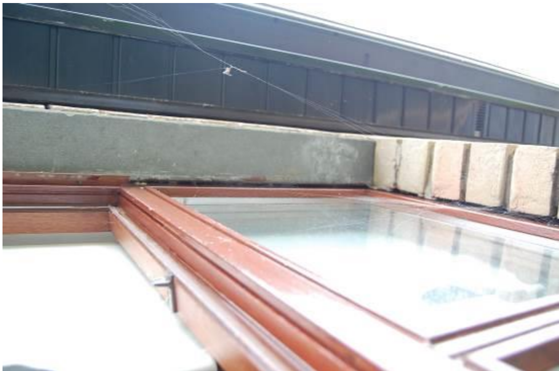
Photo 6 Missing Seal to Head and Reveal of First Floor Windows Front Elevation
