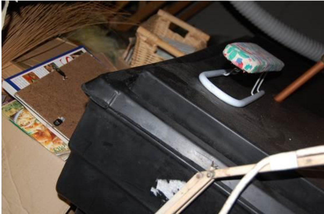
Photo 5 Water Tank in Attic Space to be Insulated
