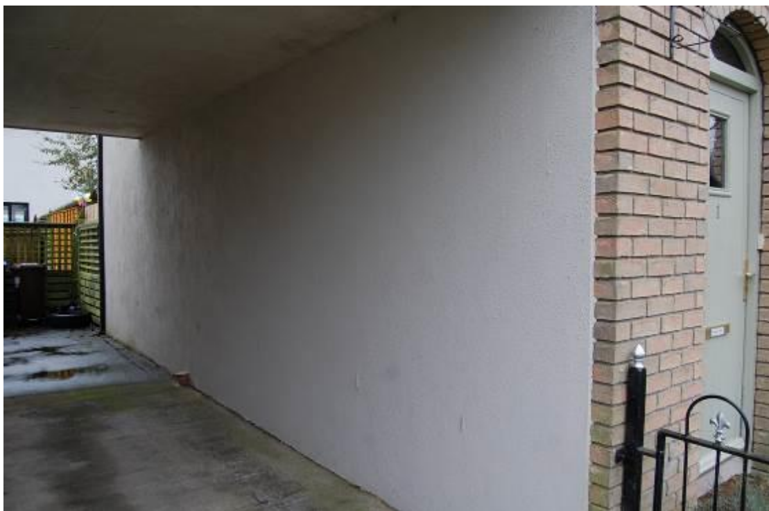
Photo 2 Side Elevation - Recommend that the ownership and rights to this area is clearly understood
