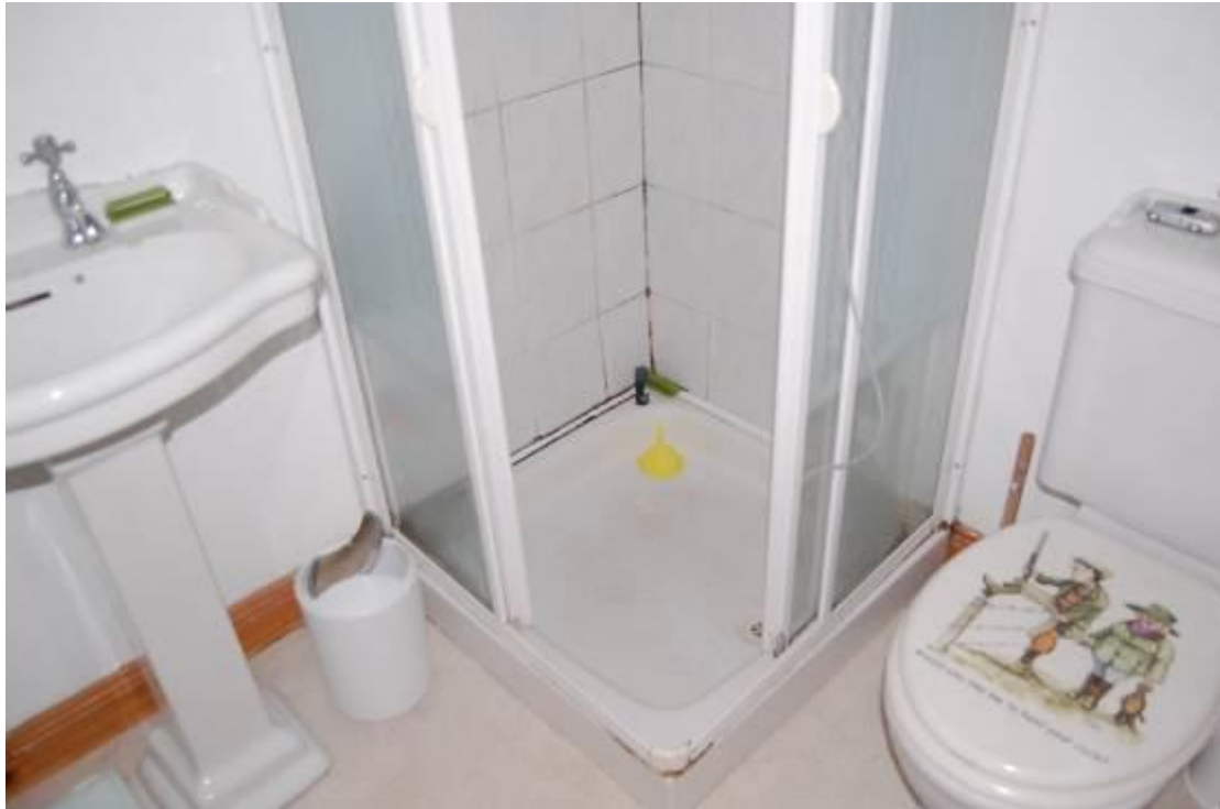
Photo 7 Tiling to Shower to be Cleaned/Replaced
