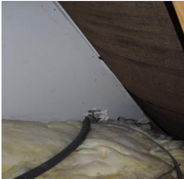
Photo 4 Hole around Water Pipe in Party Wall to be Fully Fire Stopped
