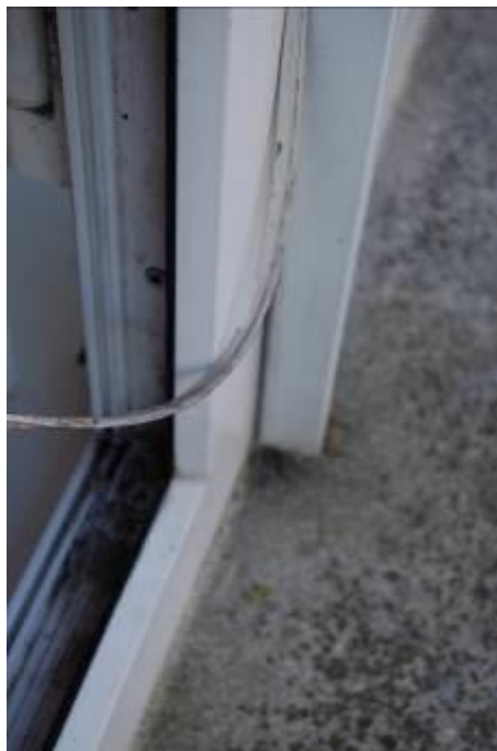
Photo 2 Seal to Window Frame Needs repair
