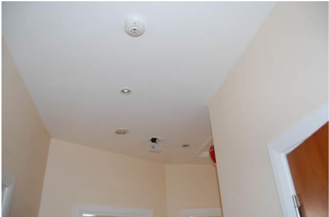
Photo 6 Apartment Fire Alarm to be Maintained
