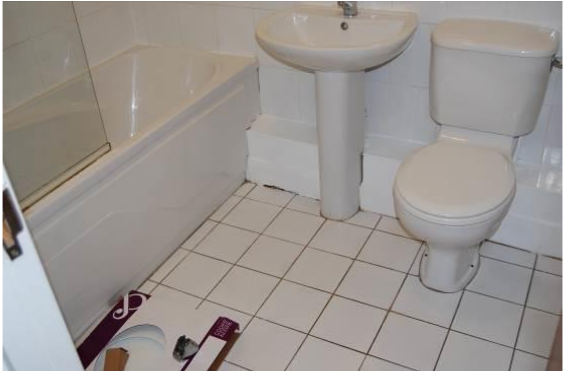
Photo 5 Tiles and Sanitary Ware need Cleaning/Upgrading
