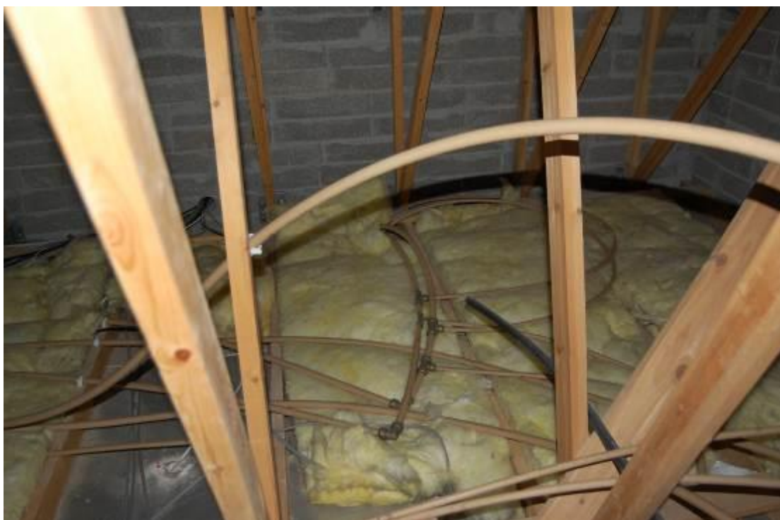
Photo 8 No Insulation to Water Pipes in Attic Space
