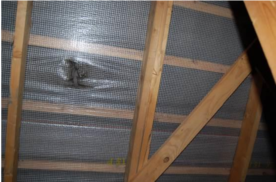
Photo 9 Tear in Felt to be Repaired
