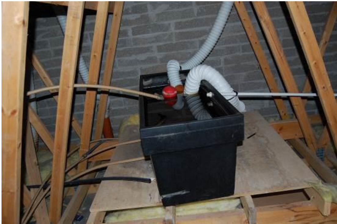
Photo 7 Ducting that has Fallen into the Water Tank and tank not Insulated
