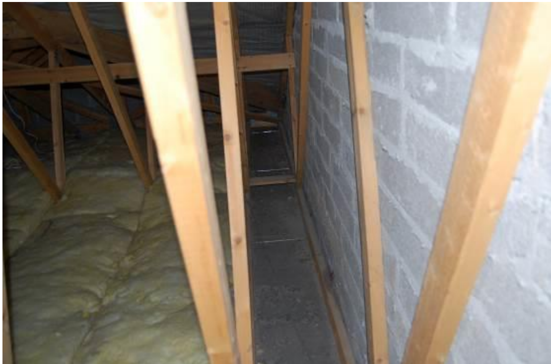
Photo 10 Strip near Party Wall with no Insulation (both sides)
