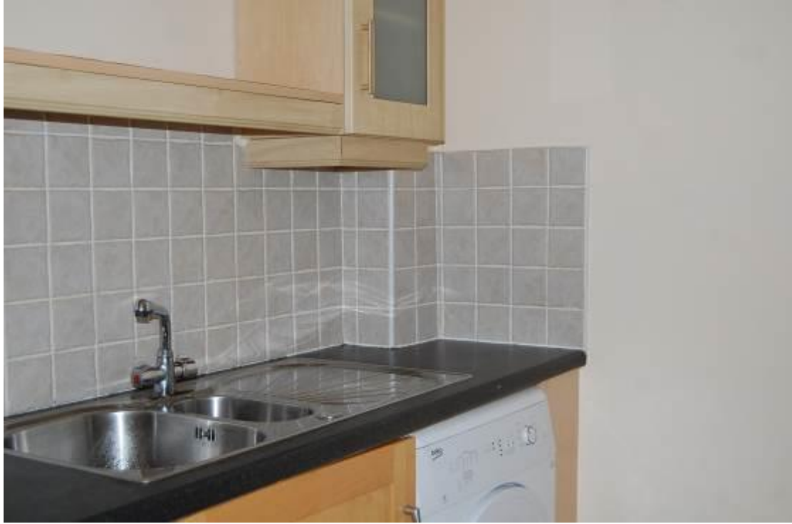
Photo 11 Boxed in Duct Pipe in Kitchen from Below
